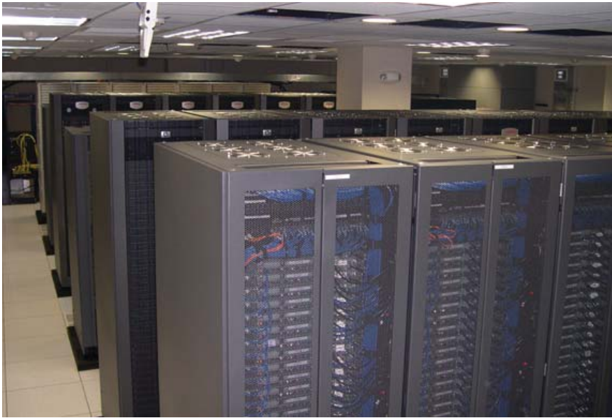
Figure 7. The Huge Server Farm at DreamWorks Animation
