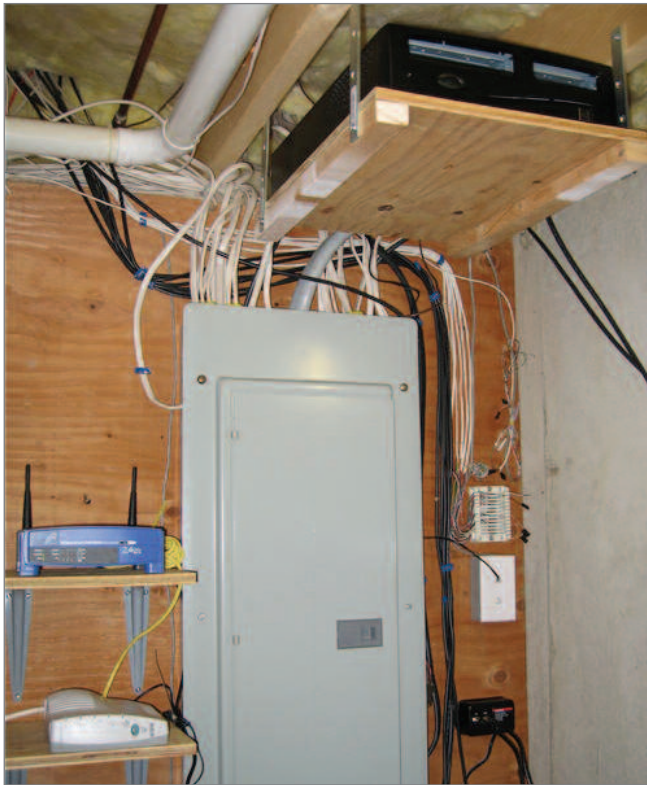
Figure 4. Skype server to provide 24/7 phone service. Server is at the top of the photo, cable modem and wireless router are to the left, and the patch board for household phone wires is to the right. In the center of the picture is the power distribution cabinet for my house.
