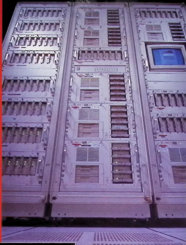
COMPAQ RACK-MOUNTED PROLIANT SERVERS
